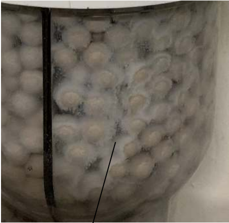
Figure 3: Salt precipitate deposited on neutralization media from Aluminum heat exchangers
